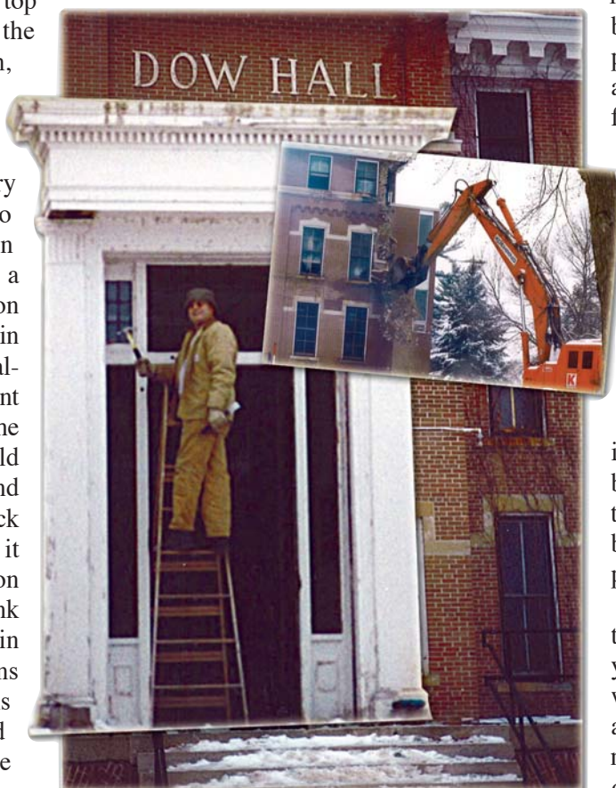
David is shown deconstructing the leaded glass windows of the Braille School's Dow Hall, a building built in the 1880s and torn down in 1998.
